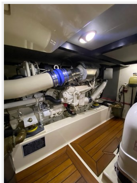
2020 Palm Beach 55 "Luce Lady" - Teak floored engine room
