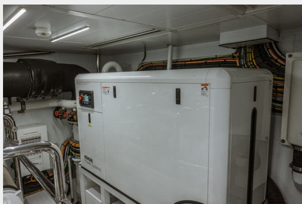
Diesel Generator Starboard
