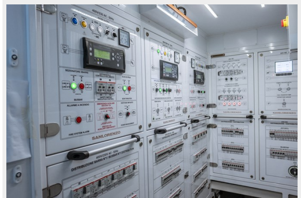
Main Electrical Switchboard
