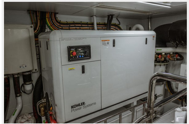
Diesel Generator Port
