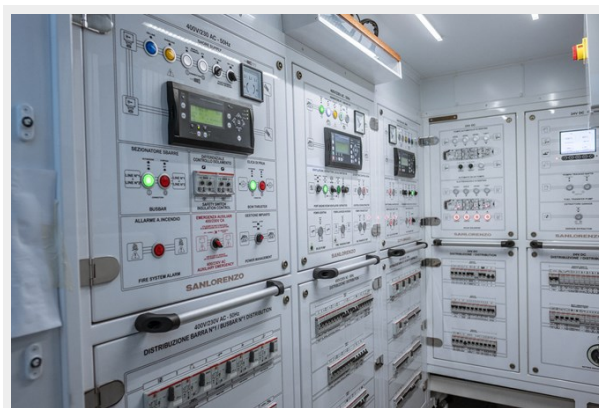
Main Electrical Switchboard
