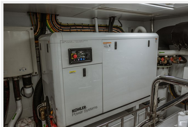
Diesel Generator Port
