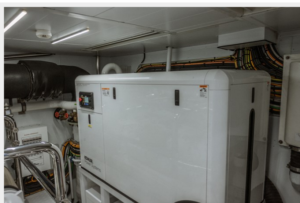
Diesel Generator Starboard
