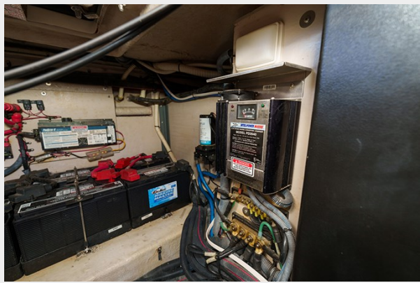
Inteli-Power PD2040 battery charger
