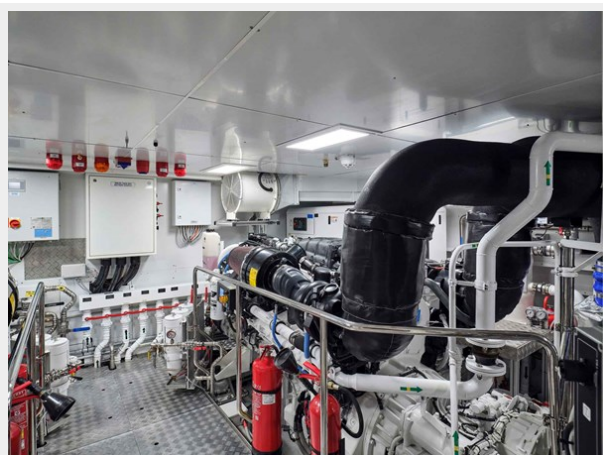
Navetta Custom Line 42 Engine Room
