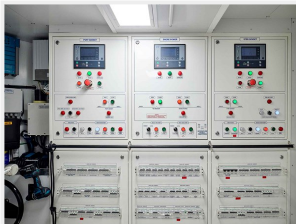
Navetta Custom Line 42 Engine Room
