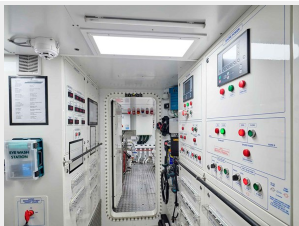
Navetta Custom Line 42 Engine Room
