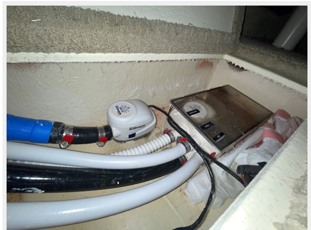
Shower Sump & Bilge
