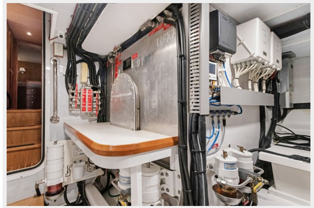
Engine room work bench fwd stbd side
