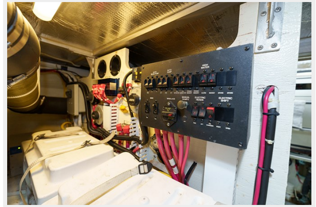
Engine room view 5
