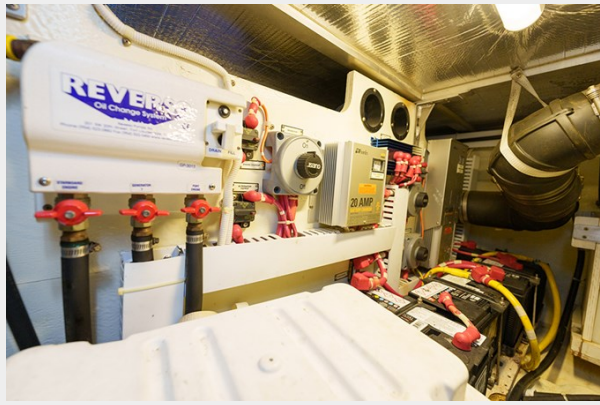
Engine room view 4
