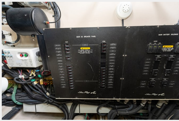
Main DC breaker panel
