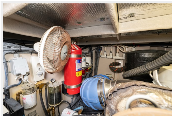
Engine room view 3
