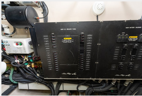
Main DC breaker panel
