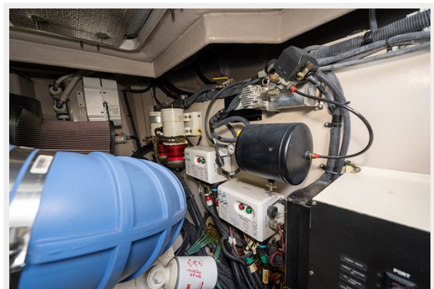
Engine room view 4
