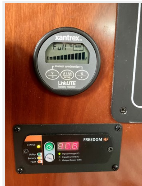
Battery monitoring system
