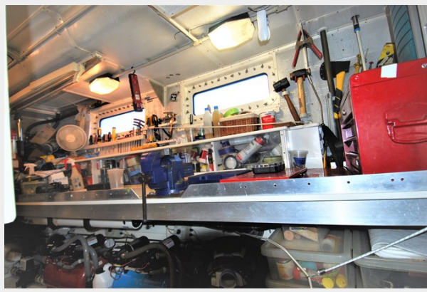
leonore - Port Engine Room
