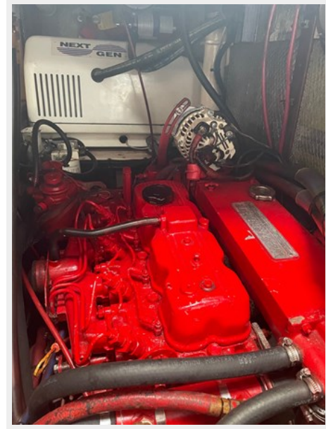
Engine and Generator
