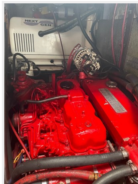
Engine and Generator
