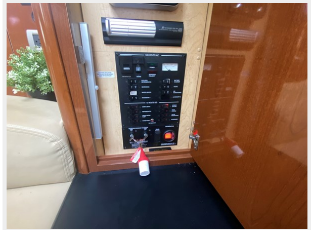
28-AC & DC CONTROL PANEL
