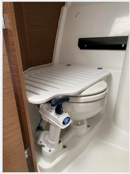
12. Marine toilet with rack down
