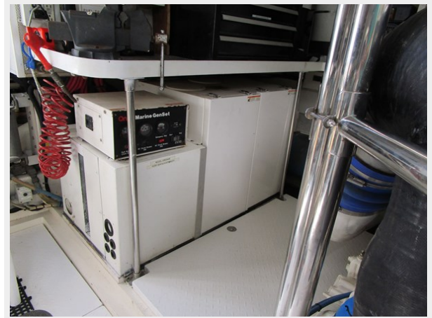
Rebuilt Port Generator
