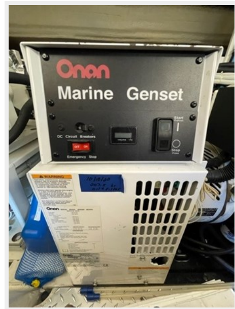
2007 TIARA 4700 SOVRAN generator control picture
