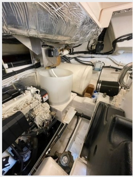
2007 TIARA 4700 SOVRAN aft engine room picture
