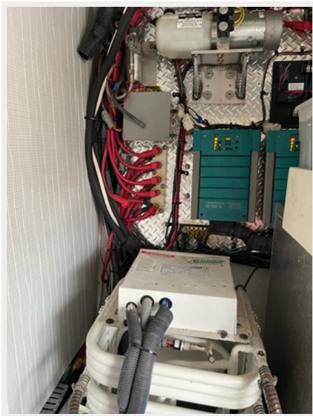
Battery charger & AC
