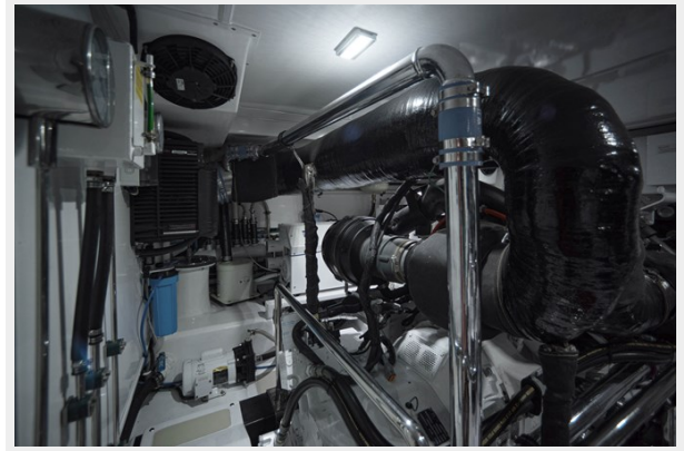
Port Engine Aft
