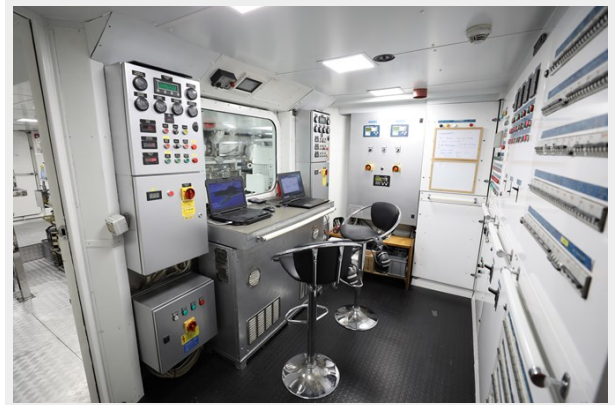
Control room TRIBU
