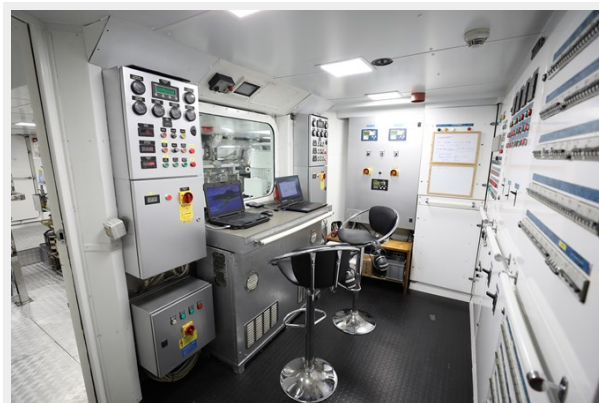
Control room TRIBU
