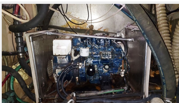
1058 Chaucer Blue Gennrator needs repair
