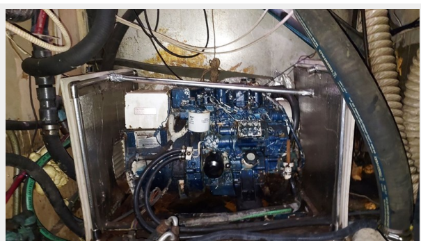
1058 Chaucer Blue Gennrator needs repair
