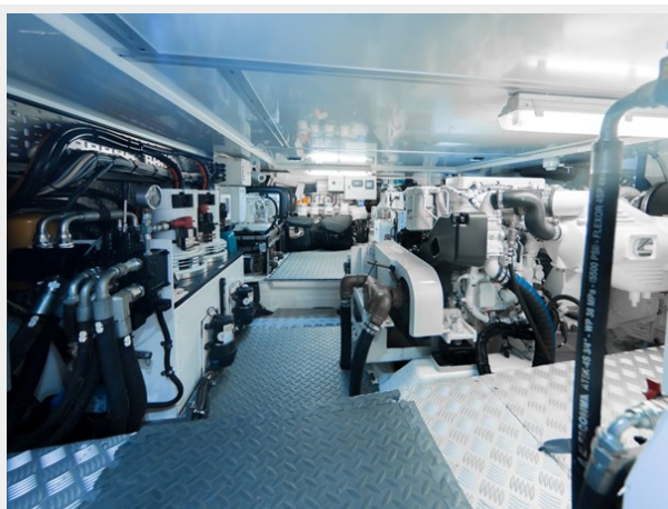
enso engine room
