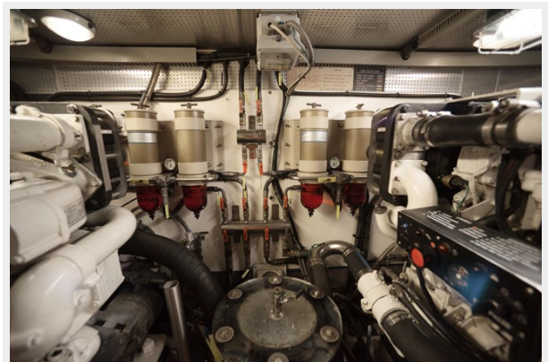
Engine Room Forward Tanks & Filters
