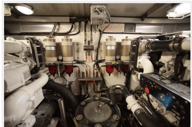
Engine Room Forward Tanks & Filters
