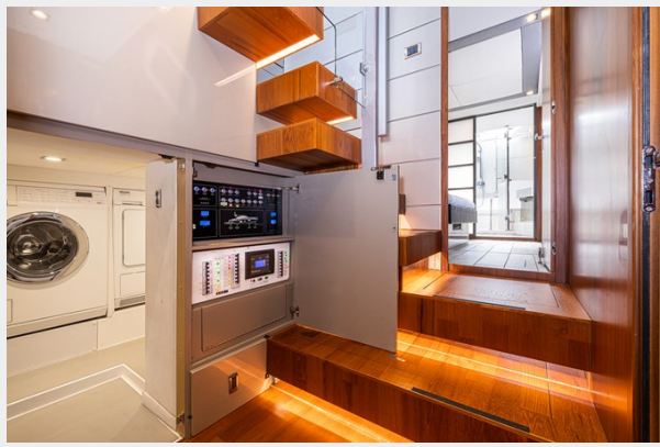
Lower Foyer showing AC Panel and Laundry
