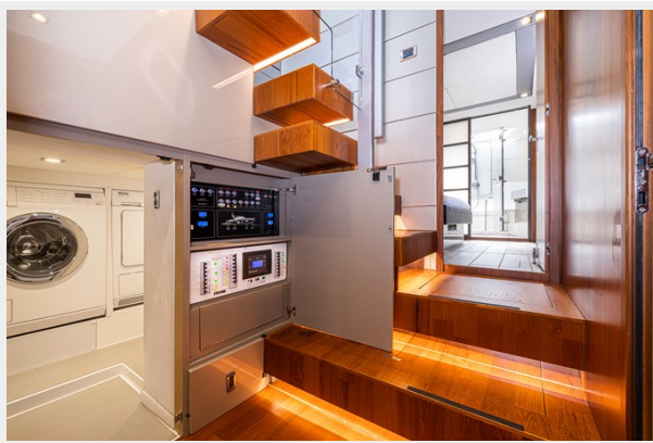
Lower Foyer showing AC Panel and Laundry
