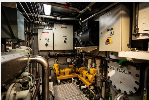
Bilge Pumps and shaft generator
