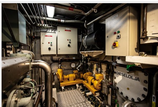
Bilge Pumps and shaft generator
