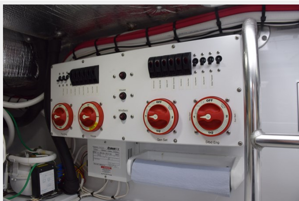
Battery Switches and Sub Panel
