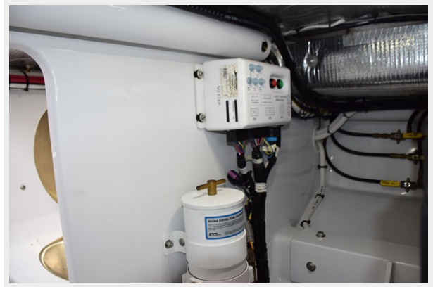
Forward Starboard Side Engine Room
