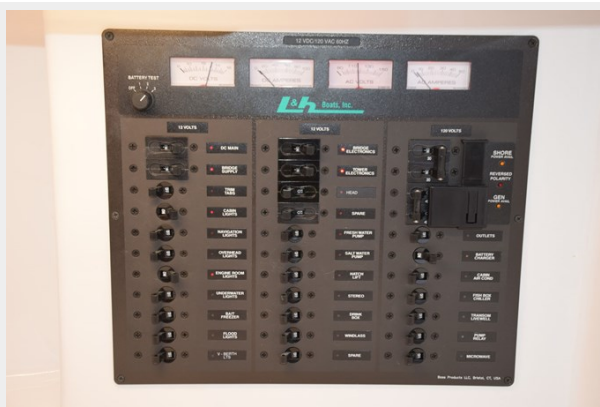
Main Electrical Panel
