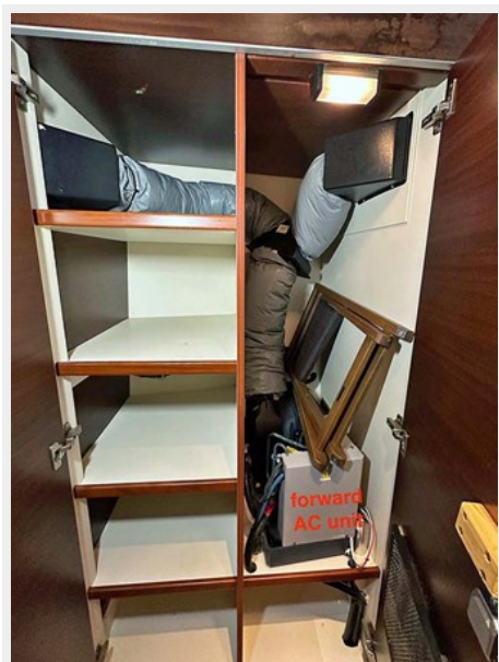
Fwd Cabin Shelving/Closet
