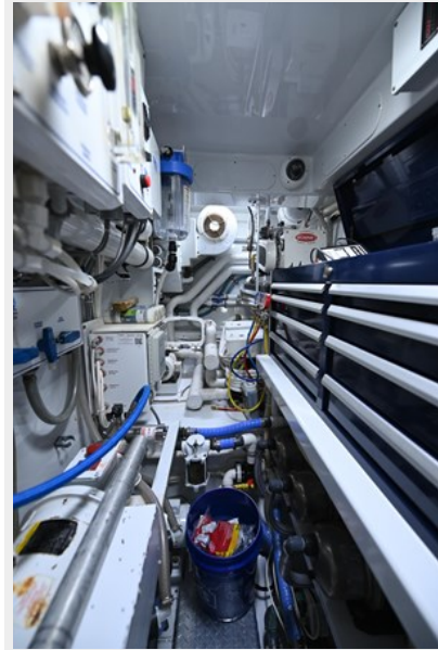
Pump Room Stb
