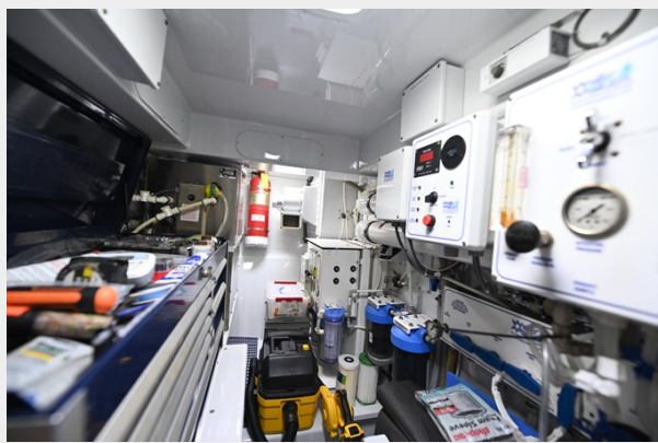
Pump Room Stb
