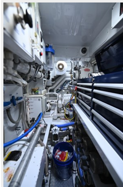
Pump Room Stb
