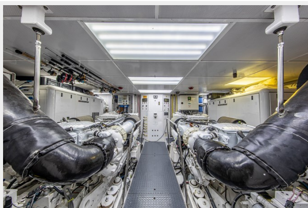
55 SPIRIT Engine Room
