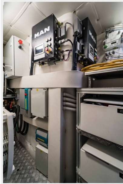
Engine room forward
