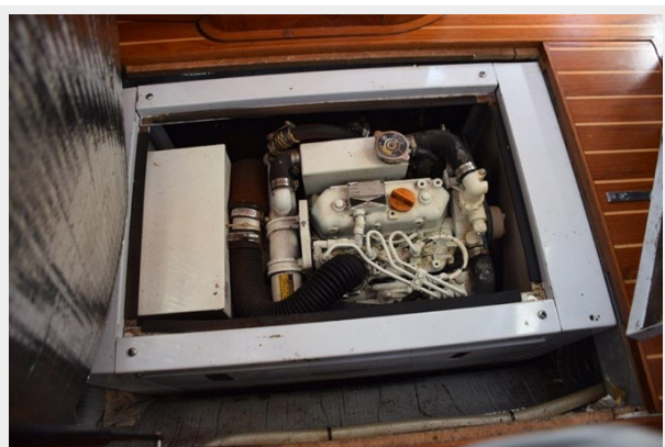
Generator in sound shield
