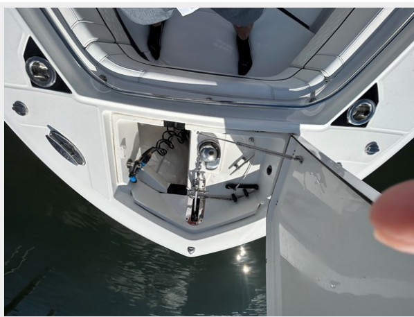
04-ANCHOR LOCKER WINDLASS & SHOWER
