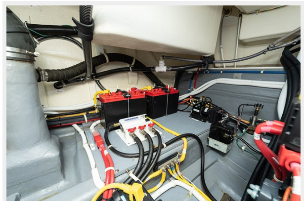
Engine room view 3
