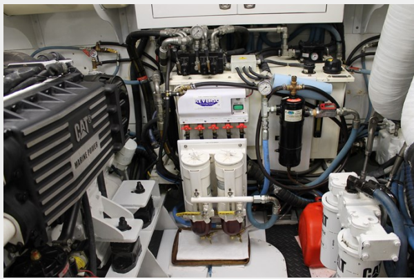
Engine Room Looking Aft
