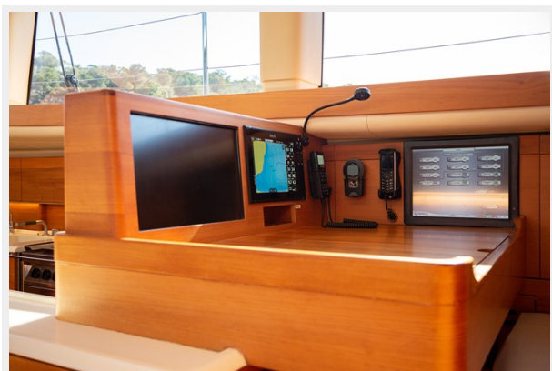
Nadejda - Navigation Station
