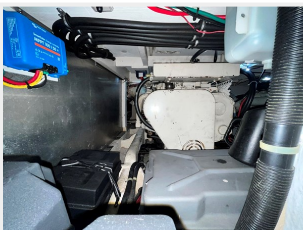
334 Engine Room Stbd
