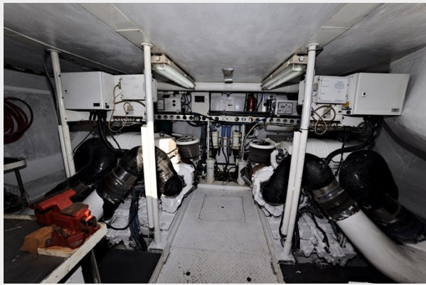
Engine Room FWD
