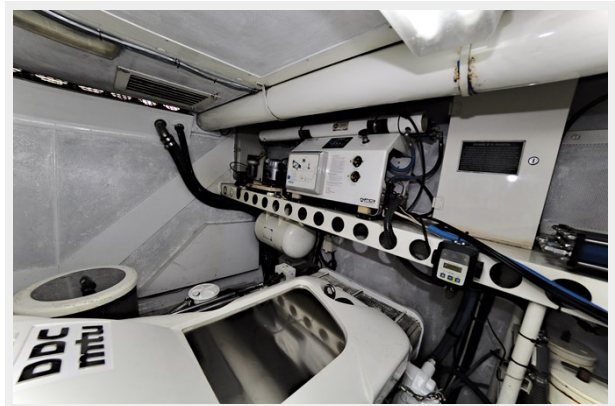
Engine Room to Fwd Port
