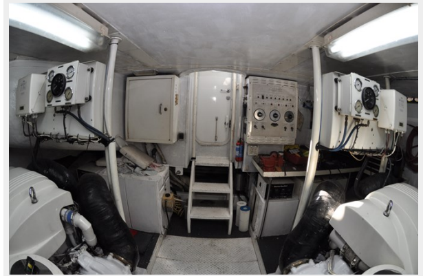
Engine Room Aft
