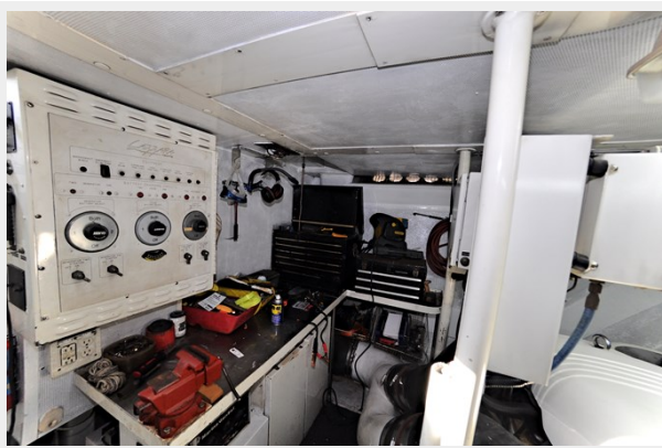
Engine Room Aft to Port
