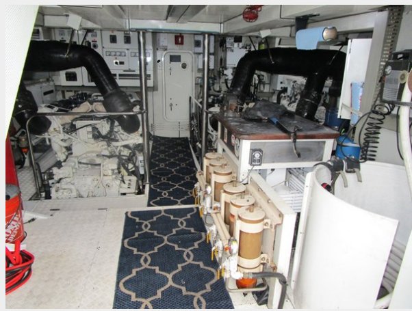
Engine Room Looking Forward
