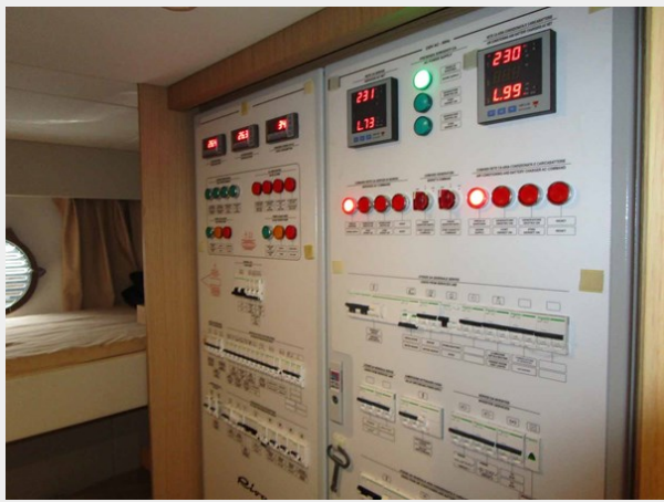
Crew Electrical Panel
