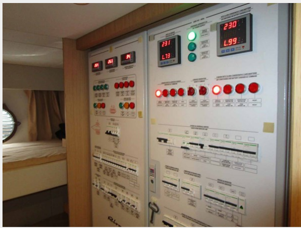
Crew Electrical Panel
