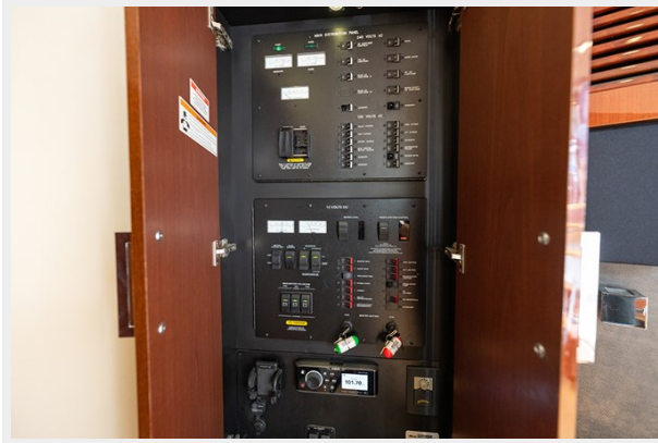
Main distribution panel
