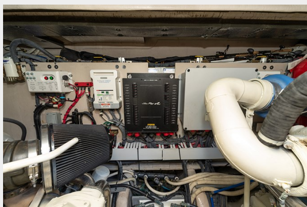
Main DC breaker panel
