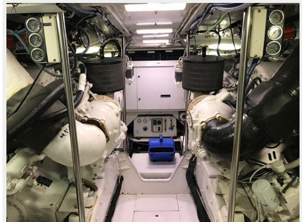
Engine Room Looking Forward
