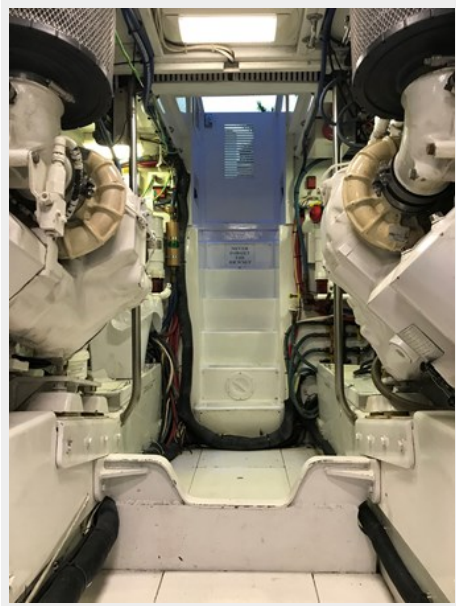
Engine Room Looking Aft
